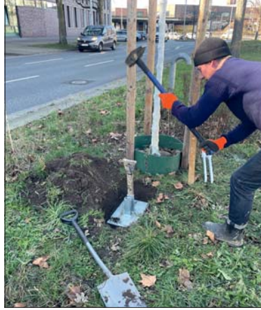
Installation des Climavi-City-Sensors in Hannover ...
